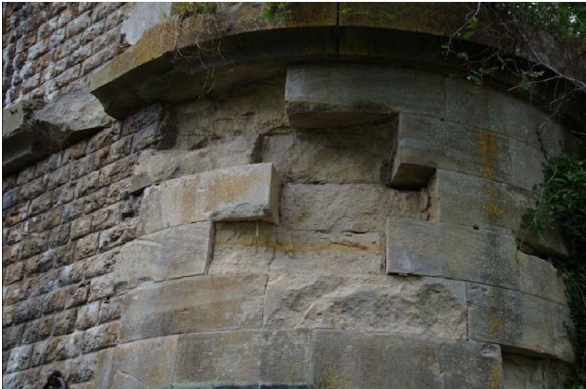
Evidence of bomb-damage still seen today on remains of the stone piers at Blois / St. Denis
